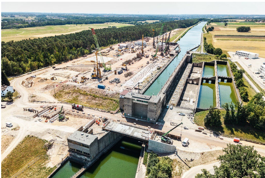
(1) The replacement of the Kriegenbrunn lock is one of the largest waterway projects in Germany.
