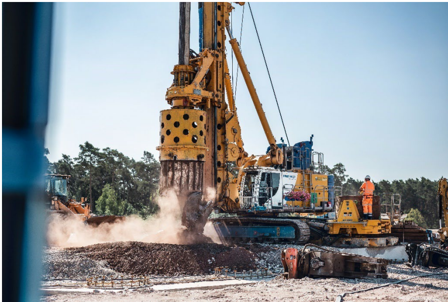
(2) Pile by pile: The retaining structure for the 30 m deep main excavation pit is constructed using the Kelly drilling method.
